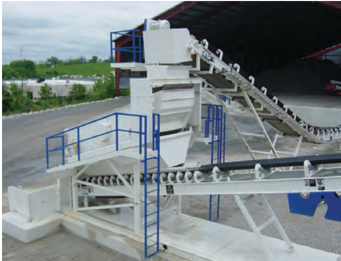
Figure 7-4. Covered Shingle Stockpile with Hard Surface Behind RAS Feeding System.
